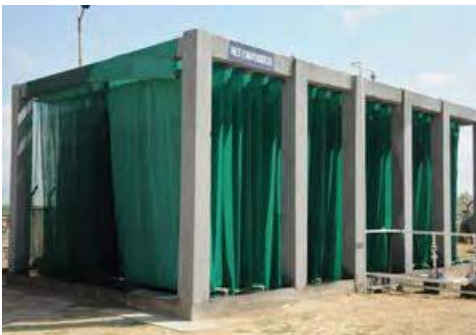
Net Evaporator for Zero liquid discharge water treatment plant
