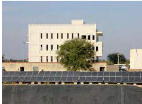
Solar Power generation to support the cause of sustainable production
