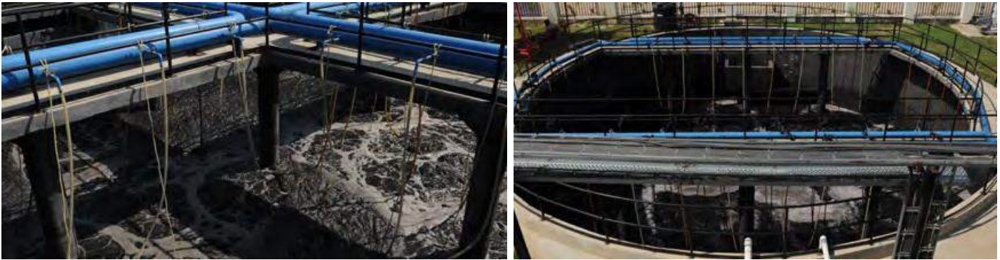
Central Effluent treatment plant for recycling dyed water
